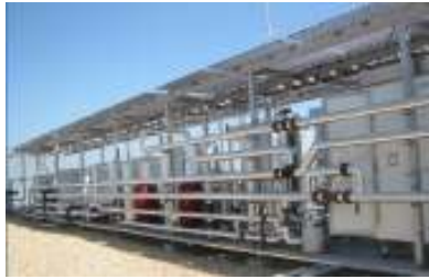
Model: LT 03 * 1 Nos Heat Source : Solar Panels
