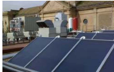
Model: LT 03 * 1 Nos Heat Source : Solar Panels
